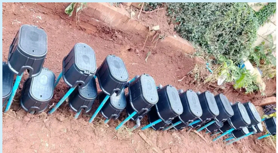
Smart City: PVC pipes and smart meters set to revamp water supply
