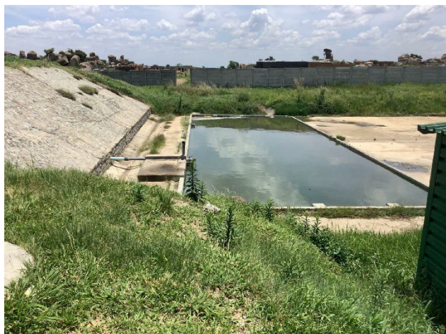
Figure 7-16: Stoneridge Wastewater sump Source: Fieldwork, December 2024
