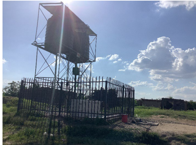
Figure 7-8: Solar powered Community Borehole
