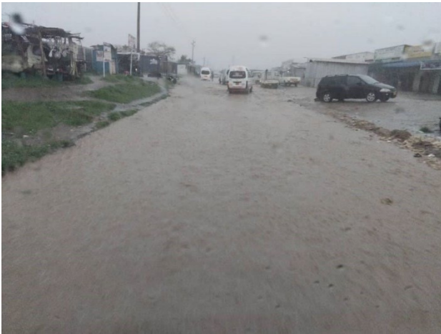
Figure 7-21:: Shoulder edge break
